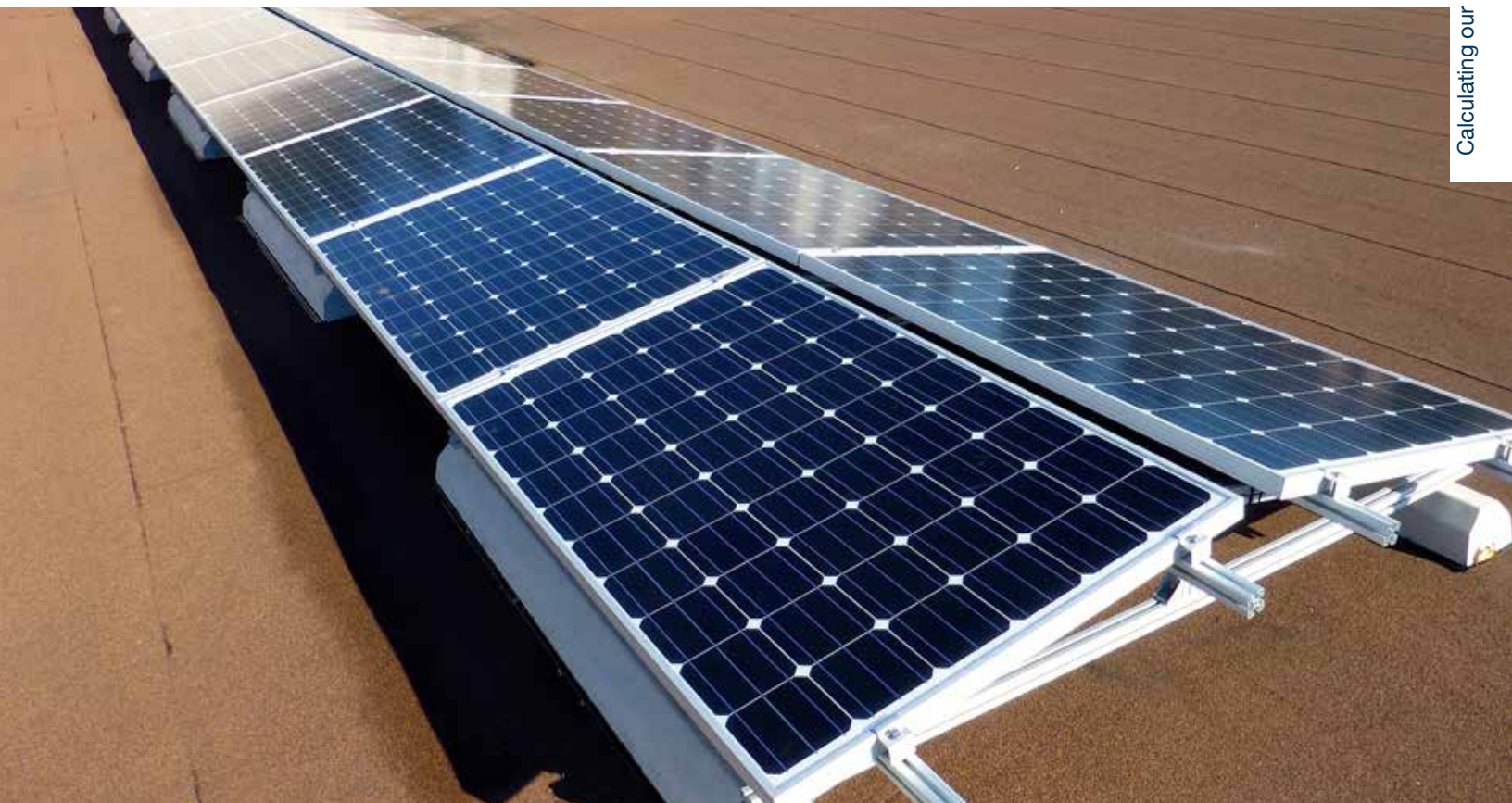
Solar photovoltaics on the Saanich Commonwealth Place
